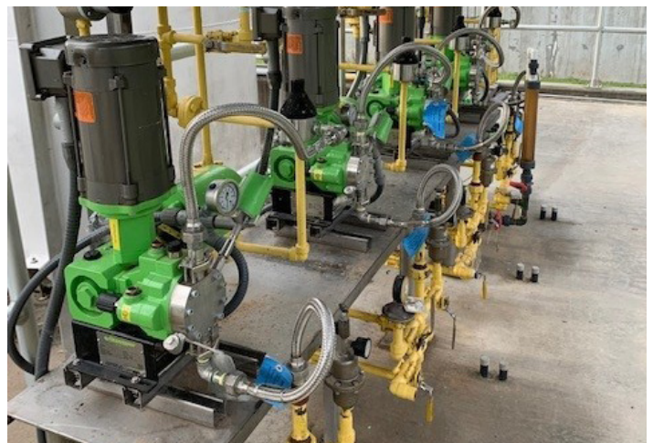
Chemical feed pumps
